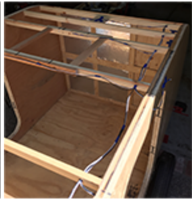
Wiring back to the galley
