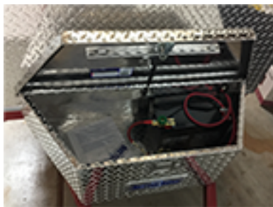
Battery box w/Battery
