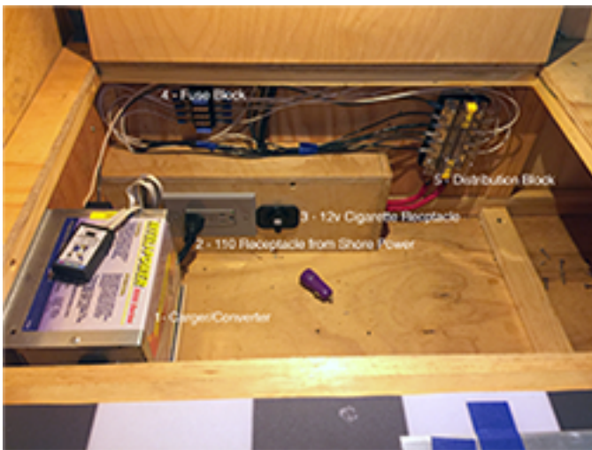
Left galley box containing all electric control
